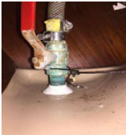
Seacock at the moment of the inspection.(Beneteau 26.5)
